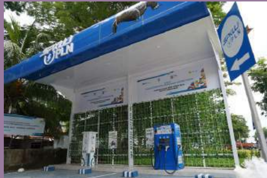
Vehicle Charging Station
